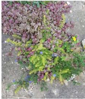
Plant concrete cracks and joints. flickr.com/photos/pdc/553335807/
